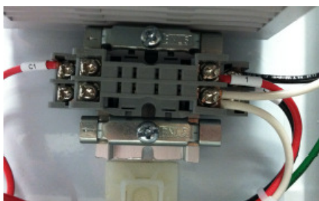
Terminal for Relay Installation
